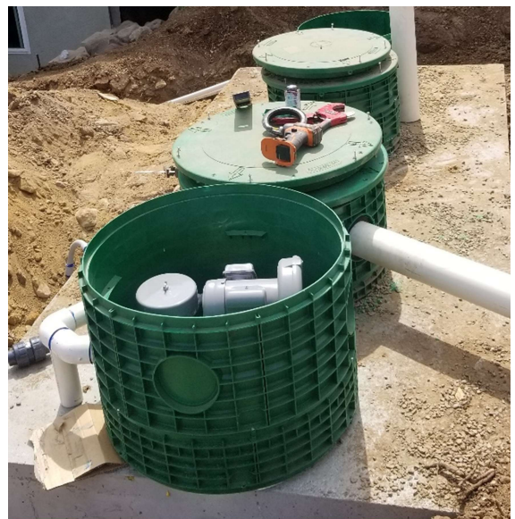
Overview with in-ground blower
