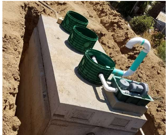
Shallow install with above-ground blower
