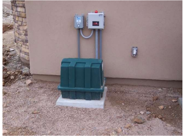
Blower doghouse on concrete w/ multiple panels
