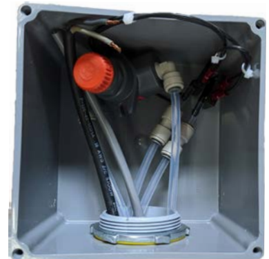
PHOTO 49 NEEDLE VALVE AND PRESSURE SWITCHES INSTALLED IN JUNCTION BOX
