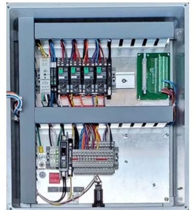
PHOTO 52 GRAVITY DISCHARGE ALARM CONTROL PANEL
