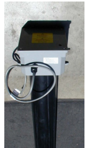
PHOTO 26 UV JUNCTION BOX ON TOP OF EXTENSION TUBE
