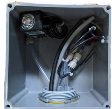
PHOTO 50 SOLENOID VALVE AND PRESSURE SWITCHES INSTALLED IN JUNCTION BOX
